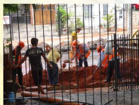
3pm the day before school started - a big hole outside the gate.
